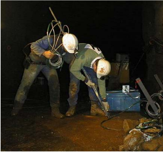
Figure 4: Photo of borehole installation frames being installed at the Tressange In-situ Test.
